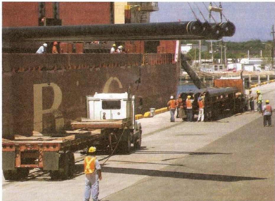
Unloading the pipes that are going to be used at the Gaseoducto project by Prepa, Codezor, the Free Trade Zone, is offering storage facilities to Skanska, the construction company for the pipeline.
